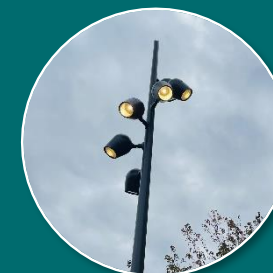
New main lighting
