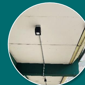
New functional lighting
